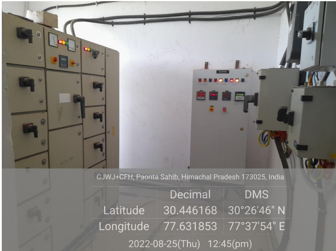
Photograph 19 Electricity Control Room Inside
