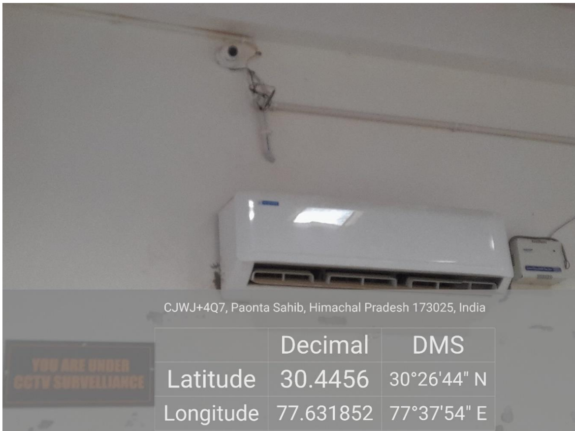
Photograph 43 ACs and Wi Fi Routers
